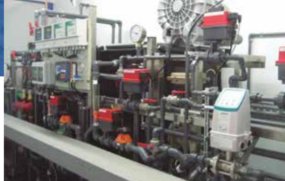
Membrane bioreactor: pilot plant
