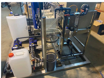
Pilot plant for drinking water treatment optimization
